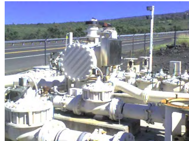
Hawaii County Dept. of Water Supply's 45-kW in-line hydro plant in Kona
