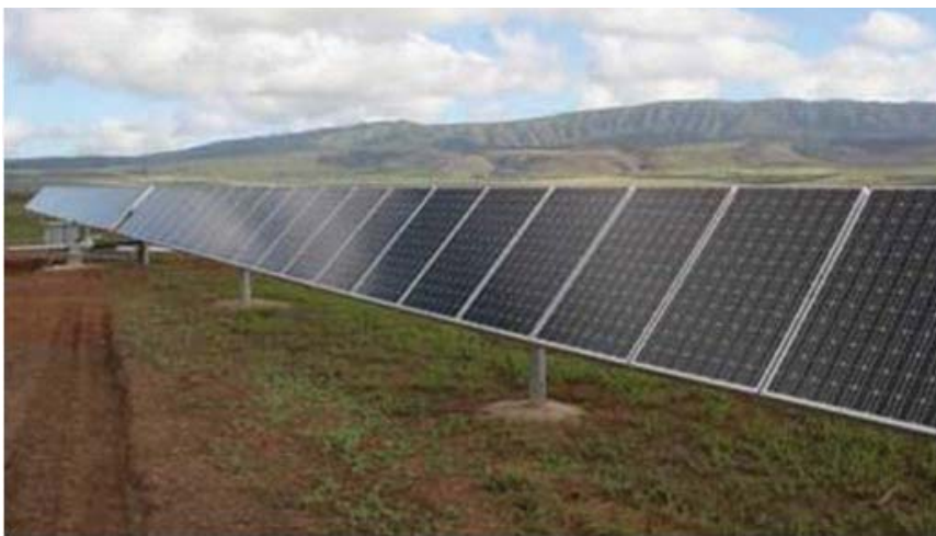
Lanai's 1.2-MW La Ola photovoltaic plant is the state's largest.
