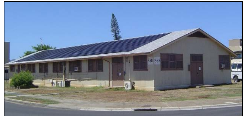
Bldg. 268 BIPV Solar Shingles 26 kW
