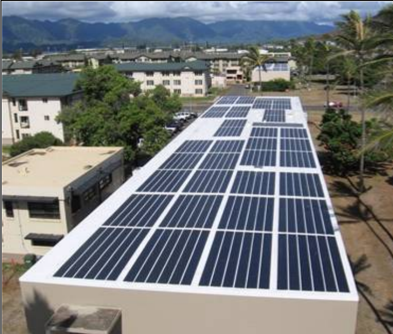
Bldg 1045 Amorphous BIPV Solar Panels (Bldgs 1033 & 1027 Similar) 32 kW Each
