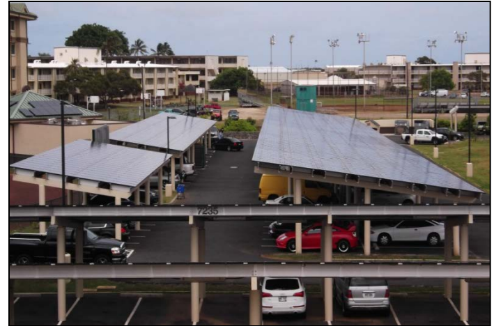
BEQ 7022 Polycrystalline Solar Carports 471 kW
