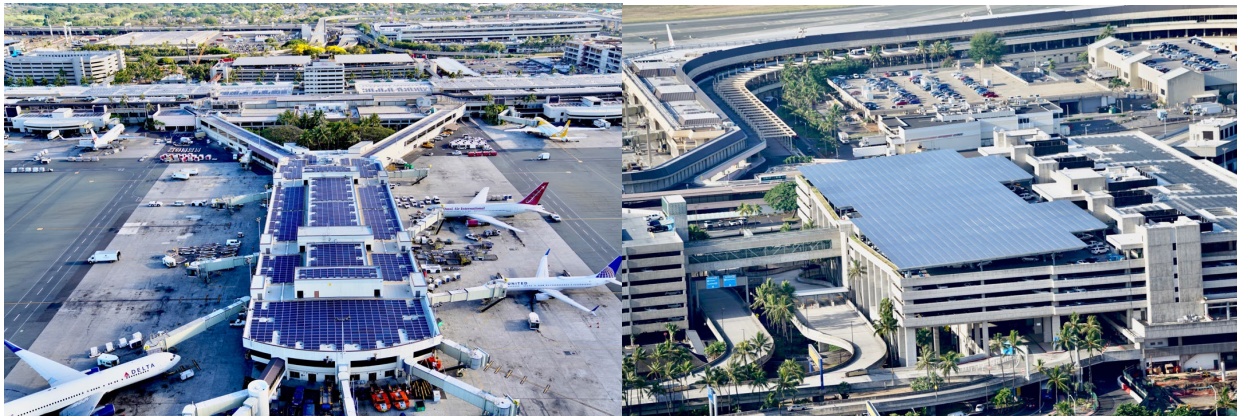
Figure 37 Solar photovoltaic panels at HNL. Image courtesy of HDOT. At the time of installation, these panels represented the single state Energy Savings Performance Contract in the nation. These panels reduce airports energy demand, but also allow for aircraft to plug-in when parked on the ramp to GPUs.
