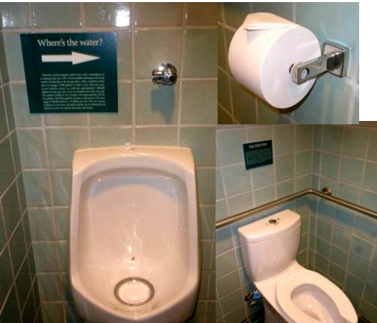
Dual flush toilet, coreless toilet paper, waterless urinal
