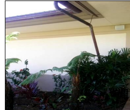
Rainwater catchment system
