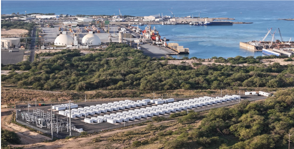
Figure 7 Plus Power Kapolei Energy Storage site. Image courtesy of Plus Power.
