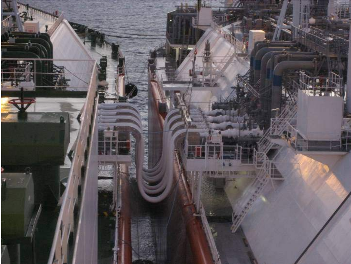
Figure 15. Ship-to-Ship Transfer via Flexible Hoses
